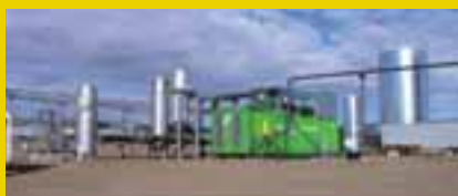
Construction of the co-generation system which turns biogas into electricity and heat.
