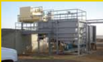
The IMUS hopper, seen here under construction, will liquefy the solid manure for anaerobic digesters.
